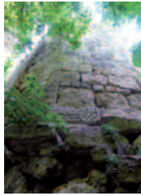
Mangup. The 2 nd defence line tower built in the early 15 th c. on the remains of the 6 th -century Byzantine walls
